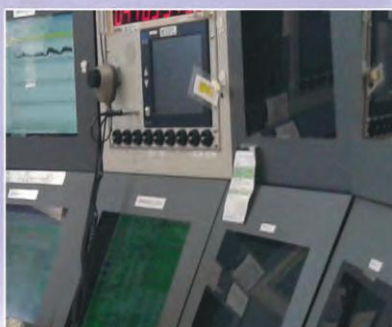
Stations Control Technology
